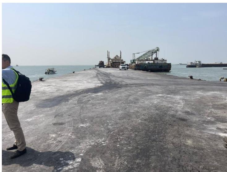
Figure 2: Quay 1: berth 1 on left/outside quay wall and berth 2 on right inside quay wall
